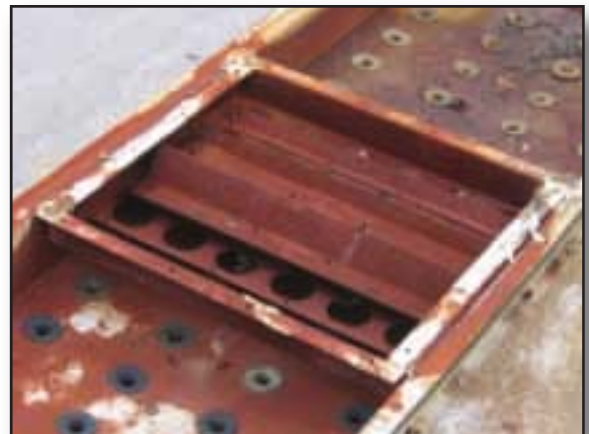
Corroded Hot Water Basin
