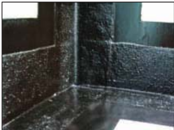
Extra Protection for Leaking Seams
