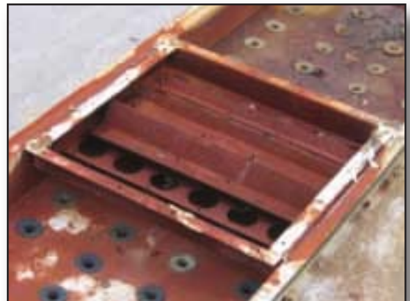
Corroded Hot Water Basin
